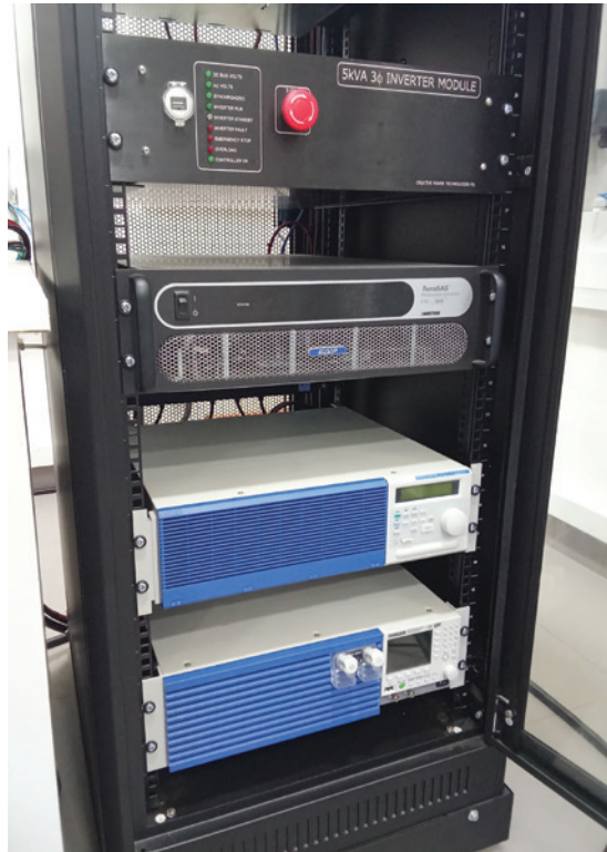
The Lanka Electricity Company (LECO)-UoM Smart Microgrid.
